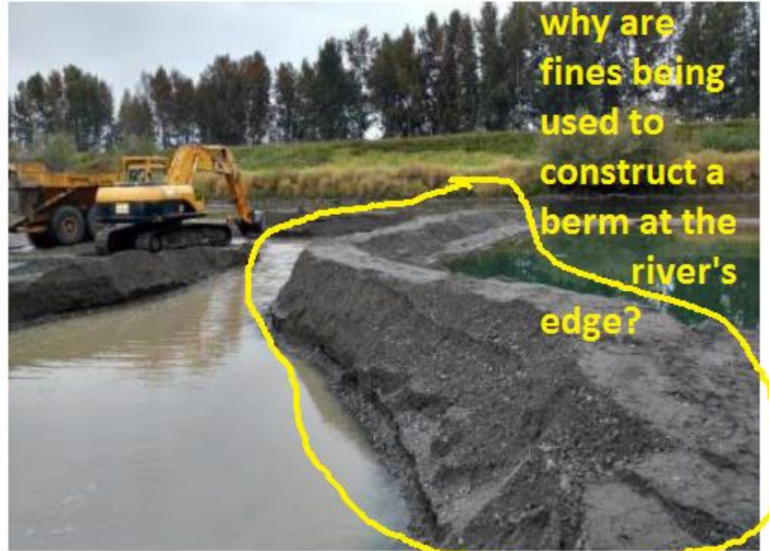
KW8: Berm constructed at upstream end and along the river to continue excavation after heavy rain. September 23, 2016.
